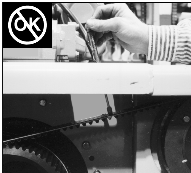
Figure 3 - 30 Tester Used Incorrectly
