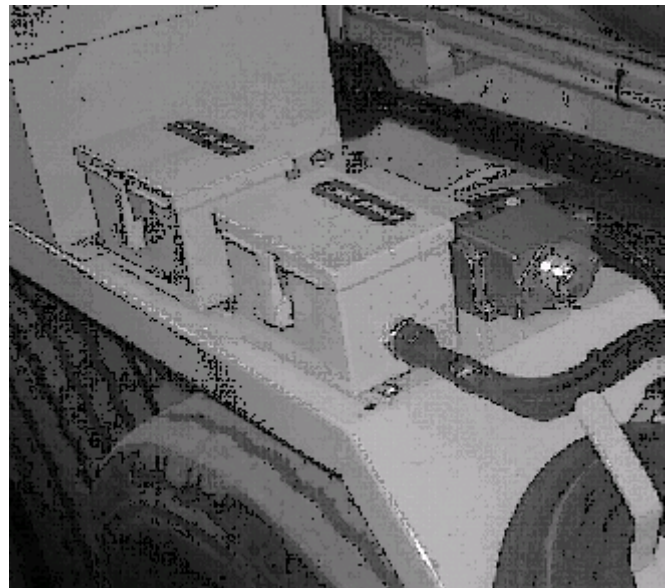
FIGURE 8 - Diesel Burners (Dual burner configuration shown)
