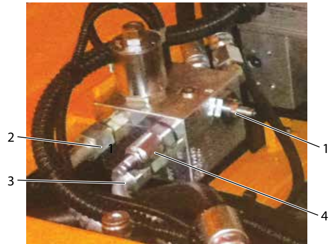
Figure 4-50. Generator Manifold Detail
