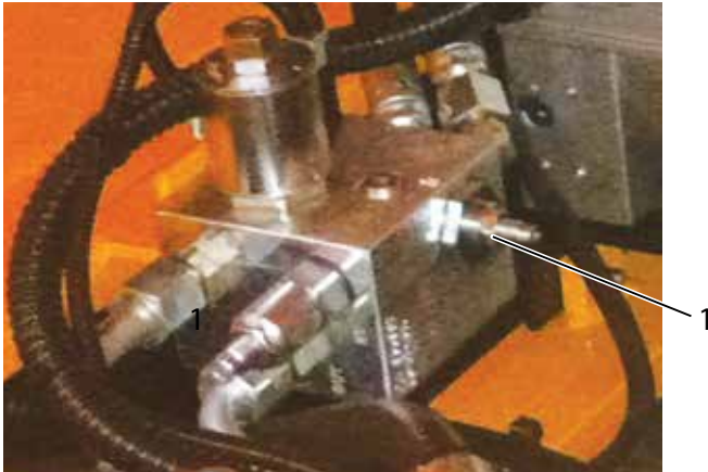
Figure 5-18. Generator Fine Tuning
