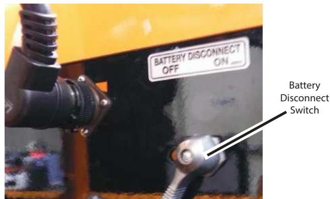
Figure 5-21. Battery Master Switch
