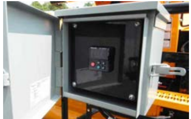
Figure 4-65. Automatic Temperature Control Box
