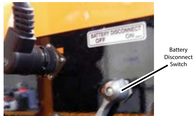
Figure 5-22. Battery Master Switch
