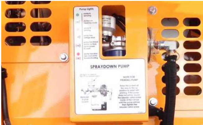
Figure 5-44. Spraydown Pump Location
