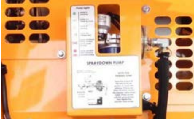
Figure 5-47. Spraydown Pump Location
